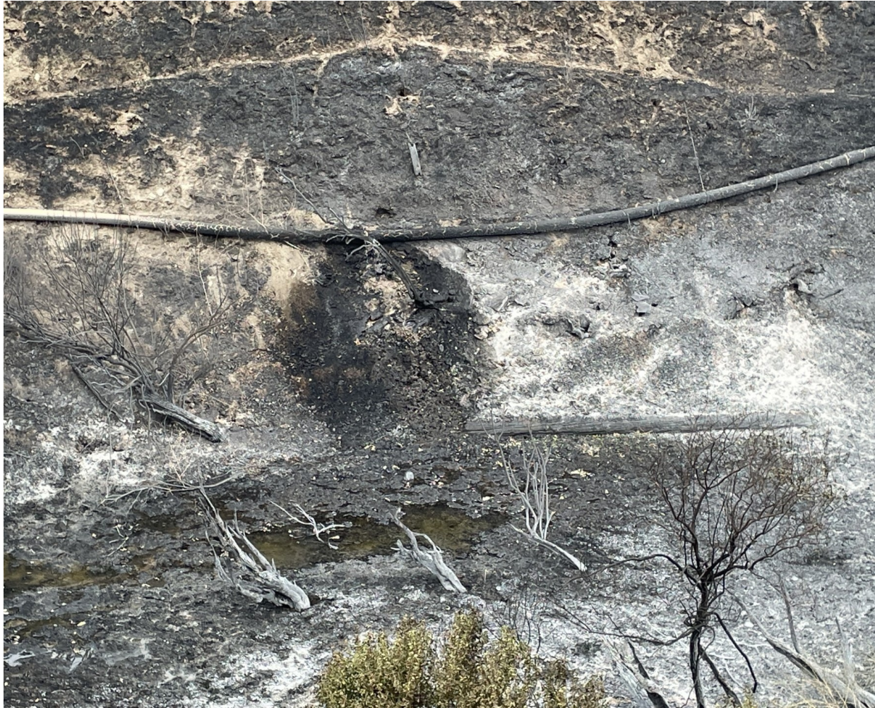
830-DISS GWTS influent pipeline.
