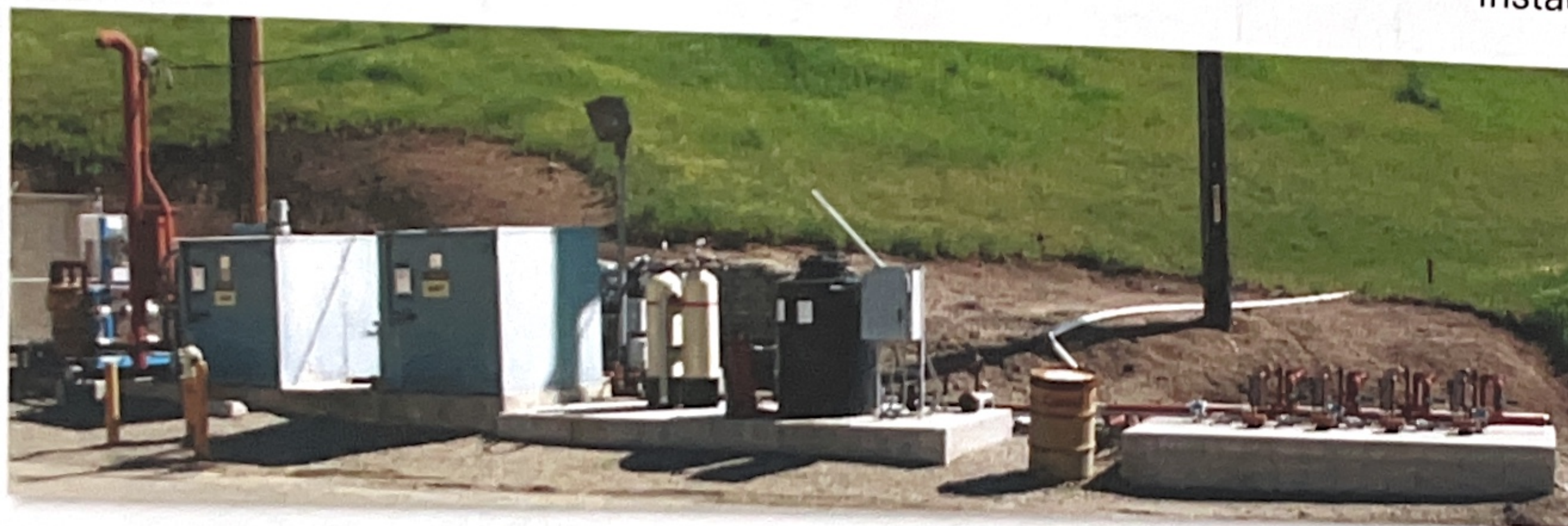
Ground water and soil vapor extraction and treatment systems reduce contaminant mass in source areas.
